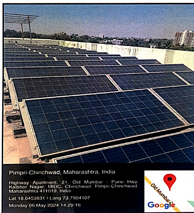
Photograph of Roof Top Solar PV Plant:
